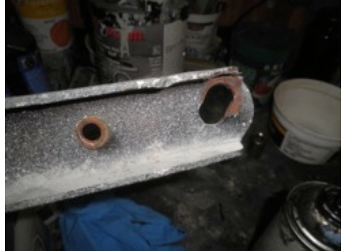
Very Oval and close to failure
